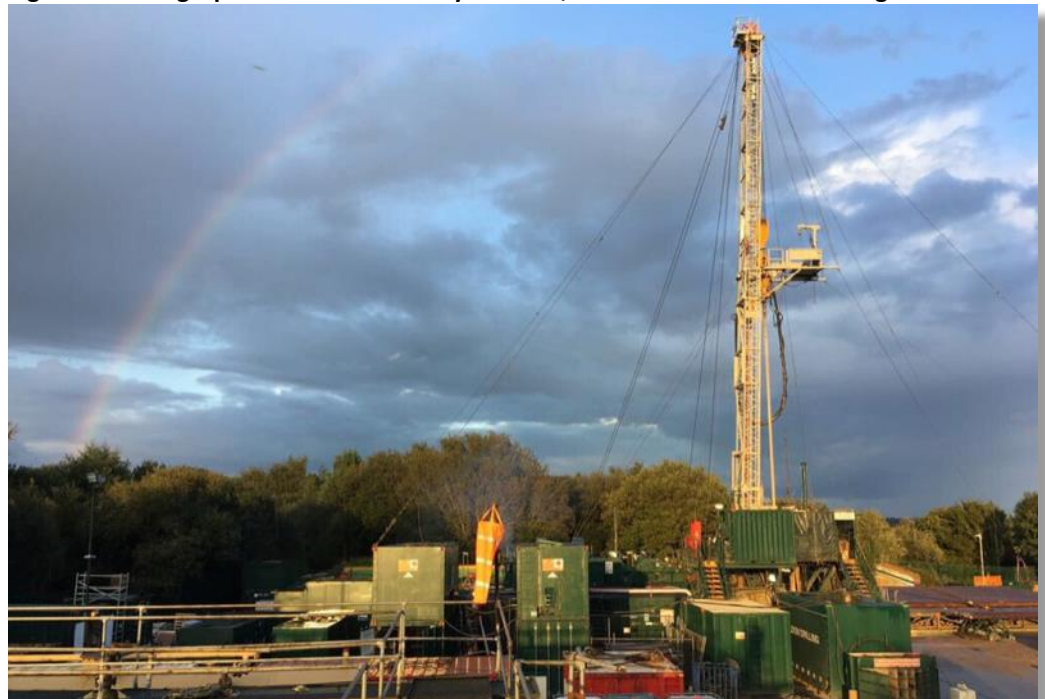
Figure 1: Drilling Operations at the Lidsey Oil Field, south of London. BDF-28 Rig.
